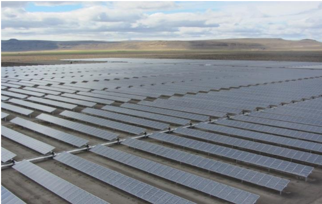
Figure 3: 5.7 MW solar installation in Christmas Valley. Photo courtesy of Obsidian Renewables.
